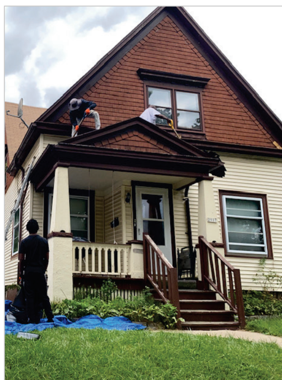
A construction team works on a roof replacement project on the Amani pilot block. (Source: Ezekiel CDC)
